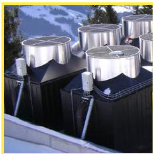
AUSTRIA SNOW MAKING PLANT
